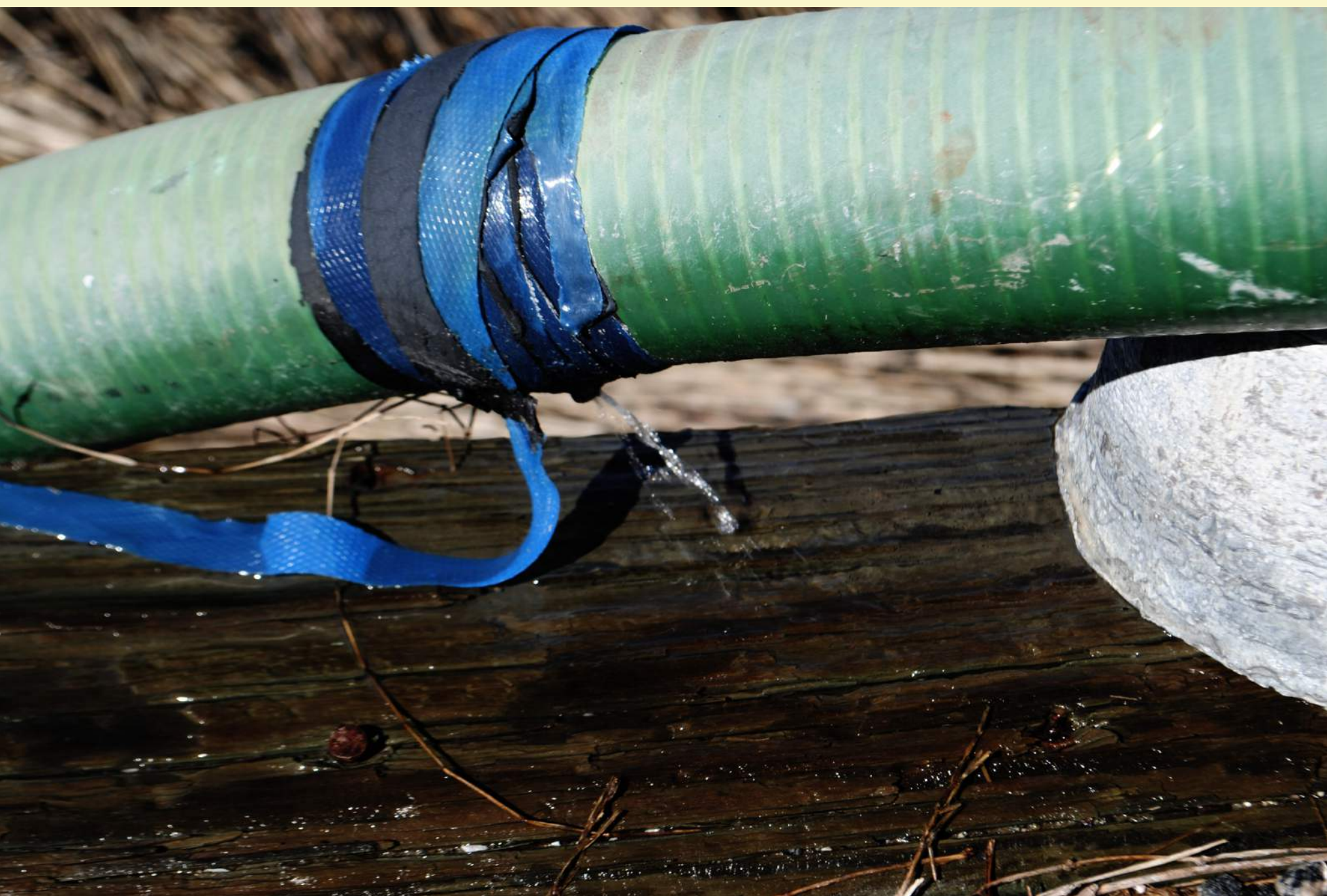
credit: Observation Finding - Pipe Leaking .
